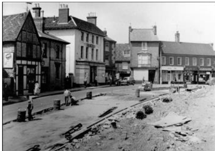
St John Street during the demolition of 1958. The large white building at the time was the Electra cinema. The old fire insurance also insured the property to the left. The cinema is now the Tickford Arcade.
